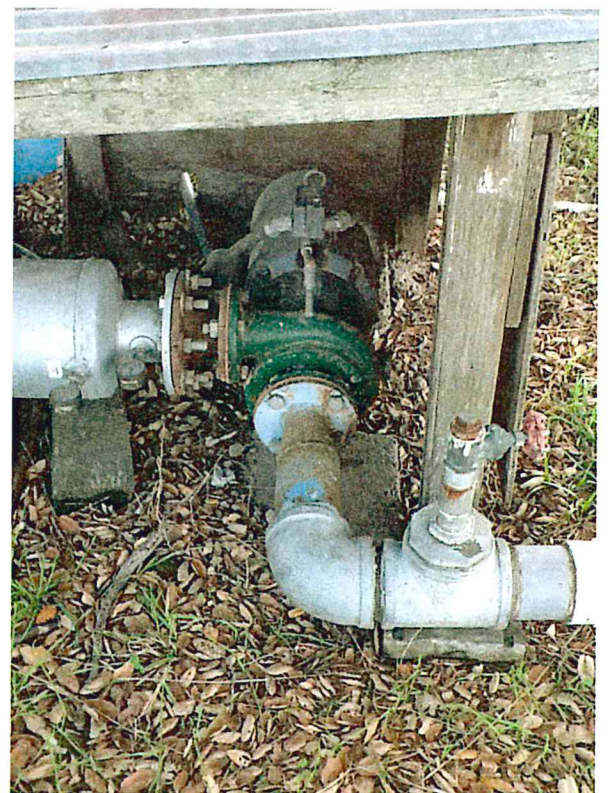
Pond Booster Pump
