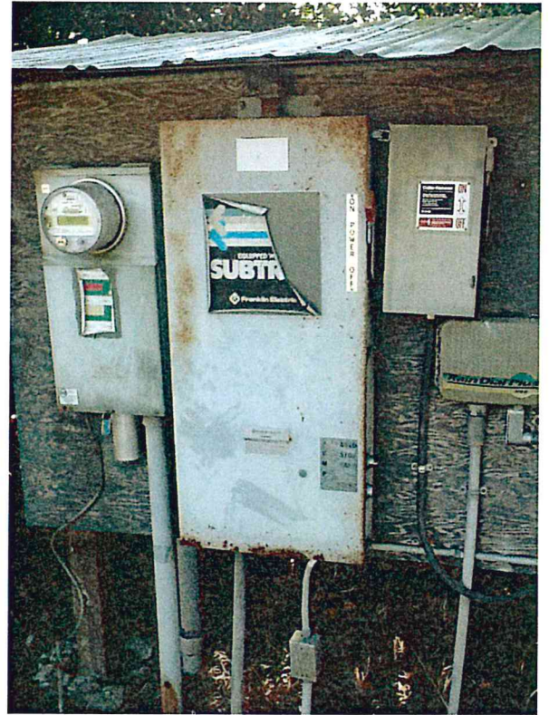
Well Pump Control Panel
