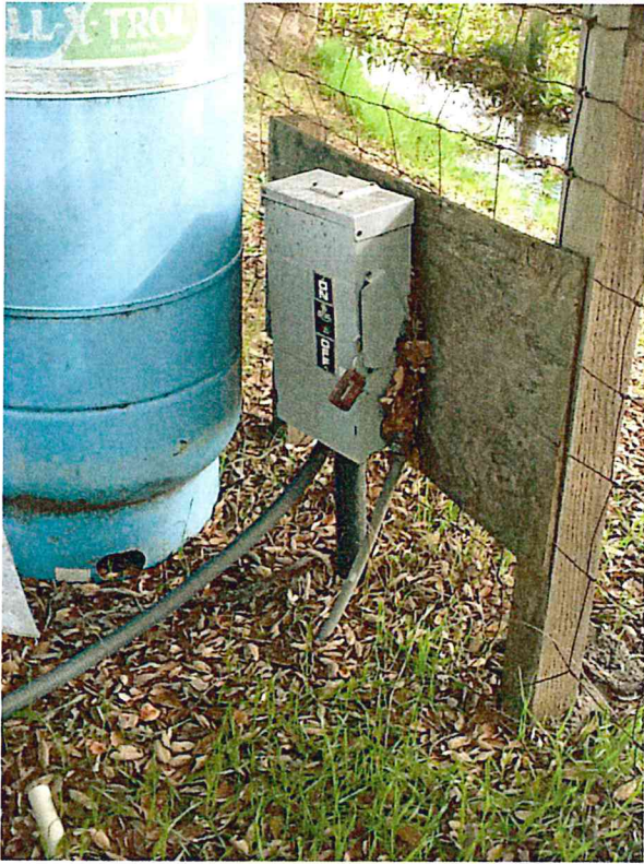
Pond Pump Disconnect
