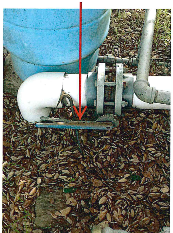
Main Shut Off Valve
