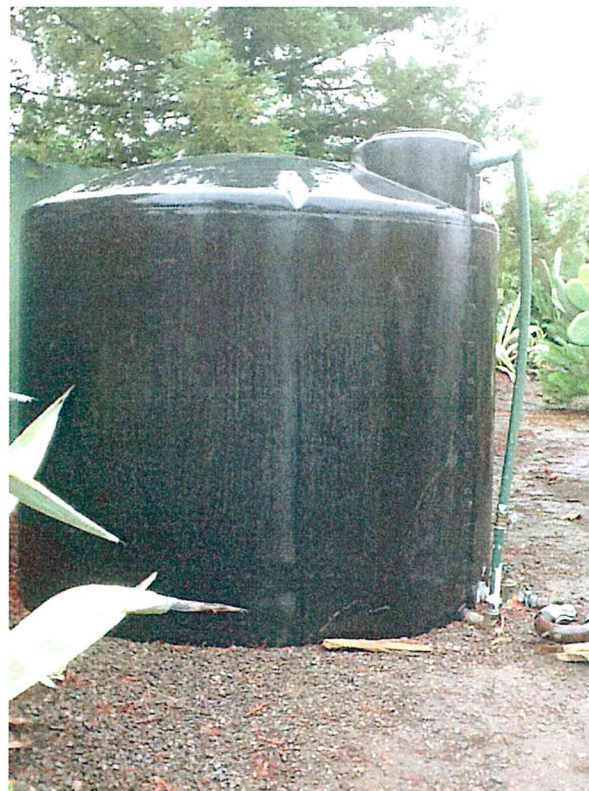
Fire Storage Tank
