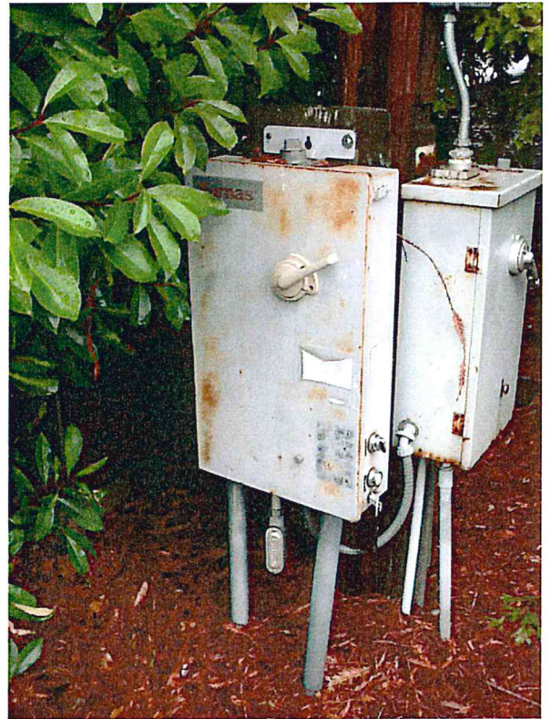
Well Pump Control Panel
