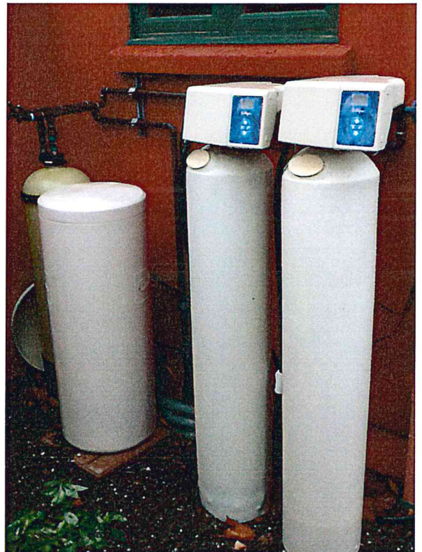
Main House Treatment System
