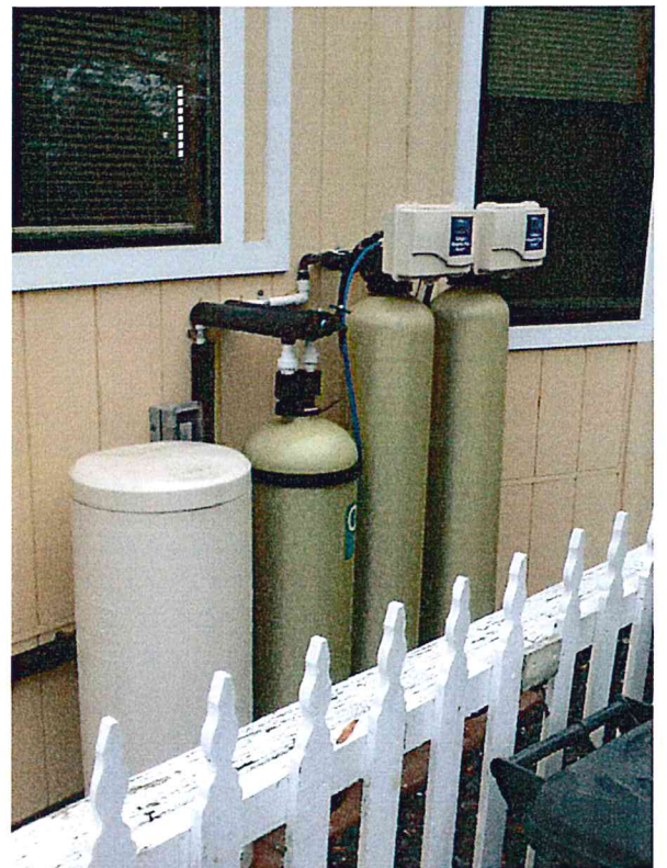
Caretaker Unit Treatment System
