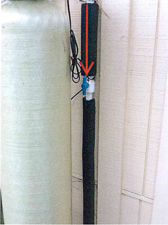
Caretaker Unit Shut Off Valve
