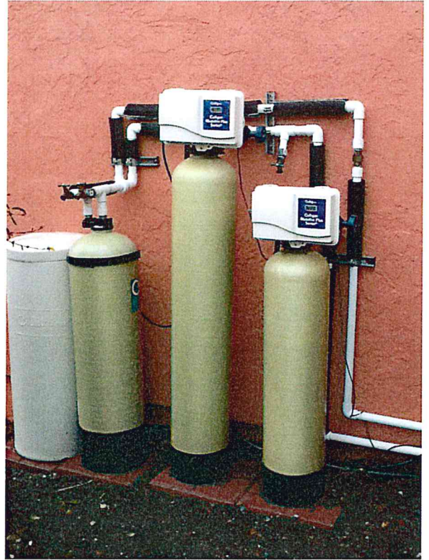
Poolhouse Treatment System
